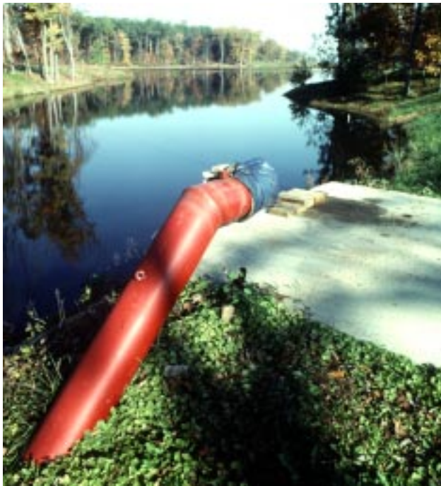
Figure 5 A dry hydrant is needed when a pond is close enough to a home or barn to furnish water for fire fighting
