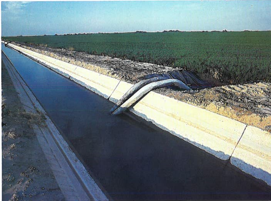
Figure 15. An irrigation water supply ditch carries snowmelt water to the fields.
