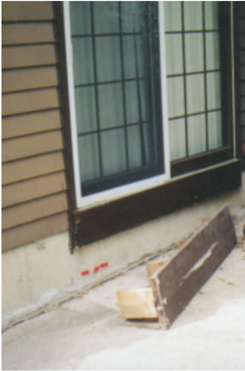
Figure 5.5: A home damaged by soil settling.
