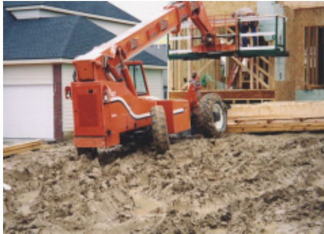
Figure 5.8: Compaction caused by the use of heavy machinery during wet periods.
