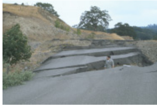
Figure 5.6: A road constructed on an unstable soil.
