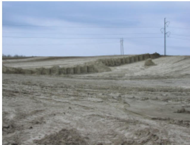
Figure 3.13: A cut on a construction site. This site is subject to wind erosion.
