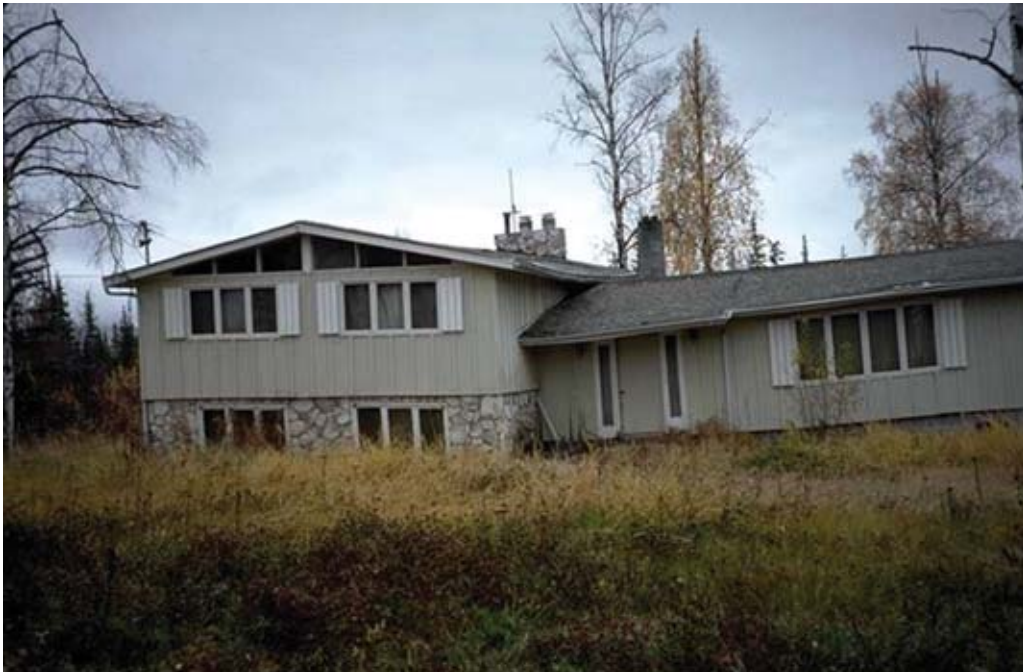
The result of building a conventional foundation on permafrost-affected soils containing massive ice. Heat transfer from the house resulted in melting of the ice and displacement of the foundation. (Photo by Alaska NRCS staff.)
