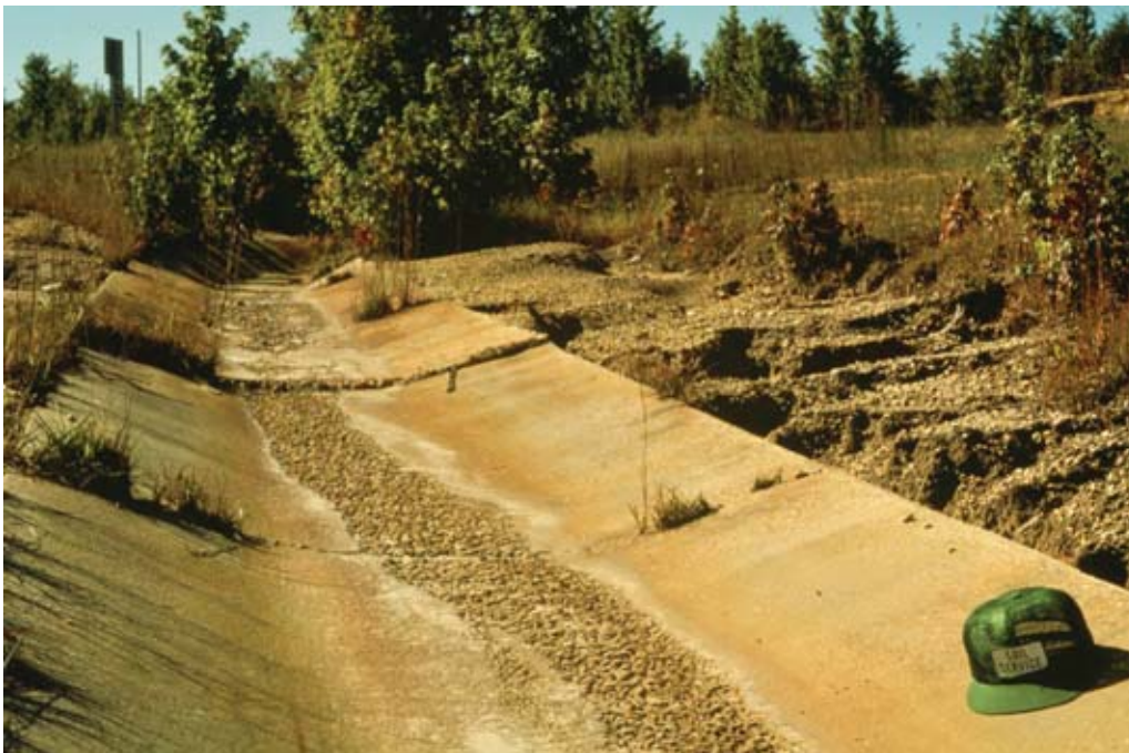
Decomposition of a concrete channel caused by acidic runoff.
