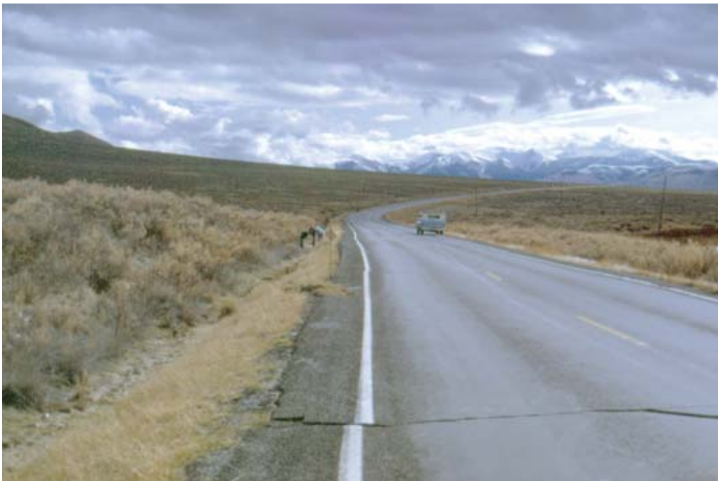
Highway offset by an earthquake fault in east-central Idaho. (Photo by Karl Hipple, USDA, NRCS.)
