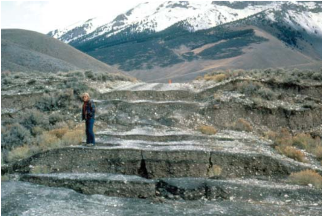
Severe road damage caused by an earthquake in east-central Idaho. (Photo by Karl Hipple, USDA, NRCS.)
